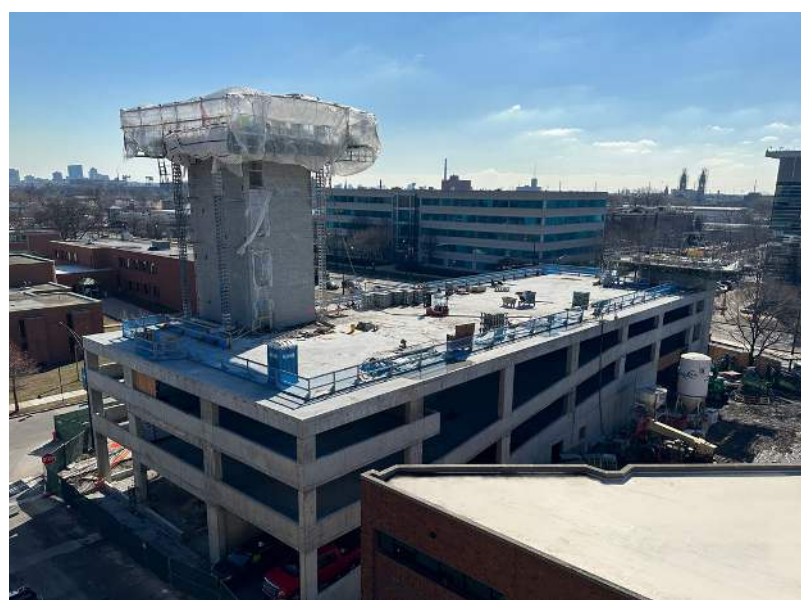
TOP: Civic, community and Lighthouse leaders break ground for The Foglia Residences at The Chicago Lighthouse. ABOVE: Eight months into construction, the building starts to take shape.
